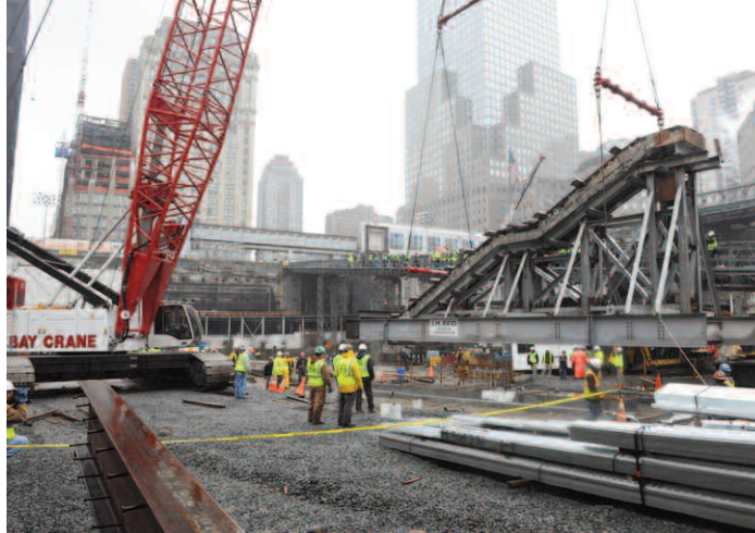
The 57-ton, 64-foot long Vesey Street stairs are lifted by crane December 12 to be rigged for a second lift to its final location.
